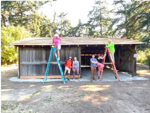
Volunteers from Michigan working on the Pratt Machine Shed. Photo courtesy of Dr. Harrison Goodall.
